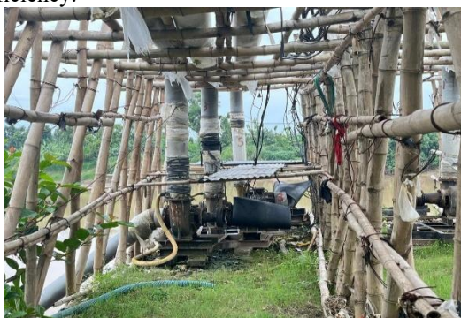
Figure 3. Irrigation Pump Infrastructure of BUMDes "Jaya Tirta"
