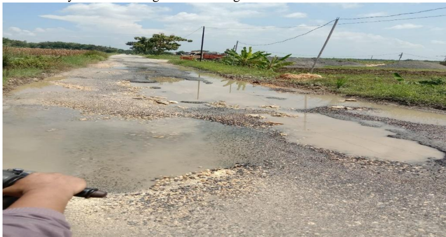
Figure 1. Road Access Damage in the Kendeng Mountains, Sukolilo District
