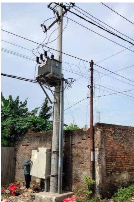
Figure 1. Distribution Transformer coded PGCE
