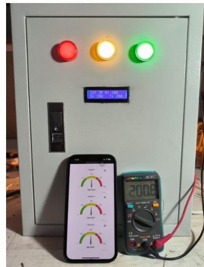
Gambar 5. Hardware Prototype Phase Failure
